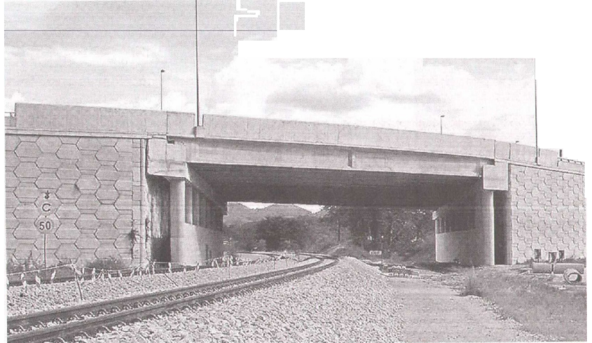
IMPRESSIVE: Nehemiah Anchored Earth Wall being applied at a cross section of a railway embankment at the MMC-Gamuda double tracking project from Rawang to Ipoh. — Bernama photo
